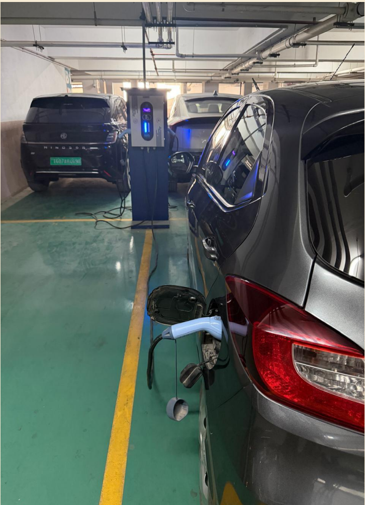
Basement SLOW CHARGER
